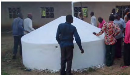
Figure 18 – Aspects of the External Plastering of the Cistern
