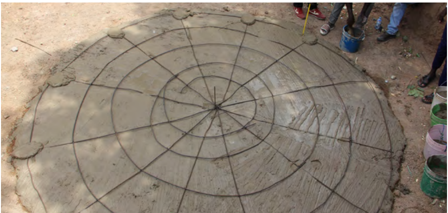
Figure 12 - Structure of the ¼' Iron Mesh at the Bottom of the Cistern
