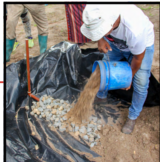
Professor Luderlândio Andrade, from UFCG, demonstrates how to set up the economic construction site in Misungwi district in November 2022. Photo: WFP
